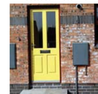
Semi-concealed Meter Box
