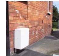
Recessed Meter Box
